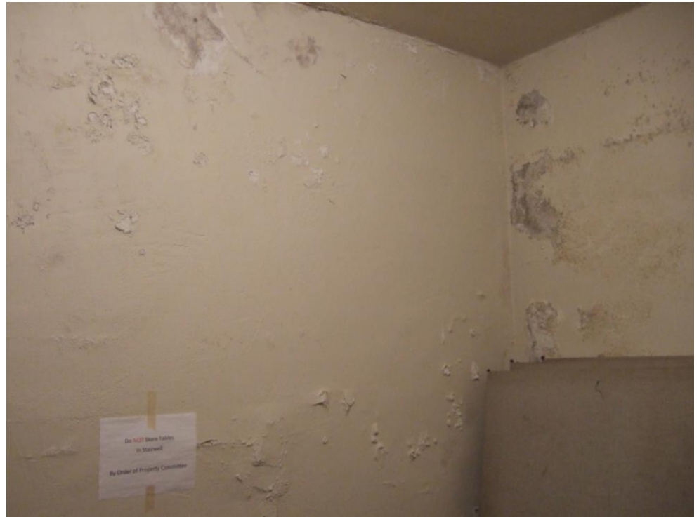
Above: Over a decade of water damage to the plaster in the northwest stairwell, basement.
