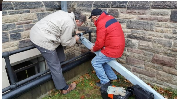
Below: David and David working on diversion of NE downpipe to carry roof water farther away from stairwell wall to
